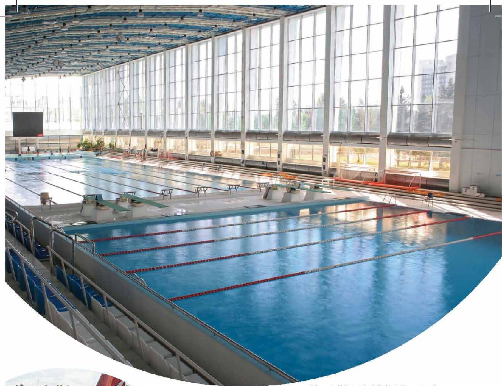
Edmonds H900 was installed in indoor swimming centres to reduce condensation and humidity.
